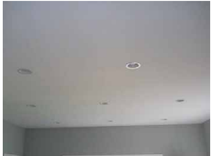
Recessed can lighting
