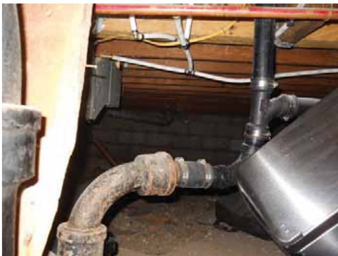
Waste piping at crawl space
