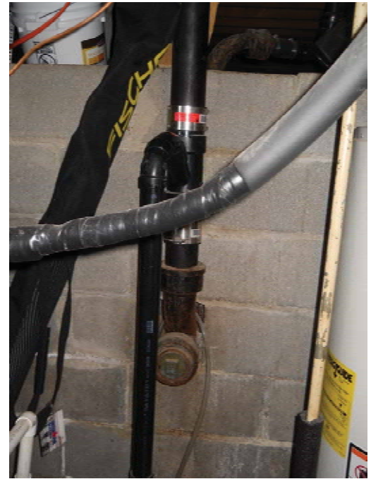
Waste piping at basement.
