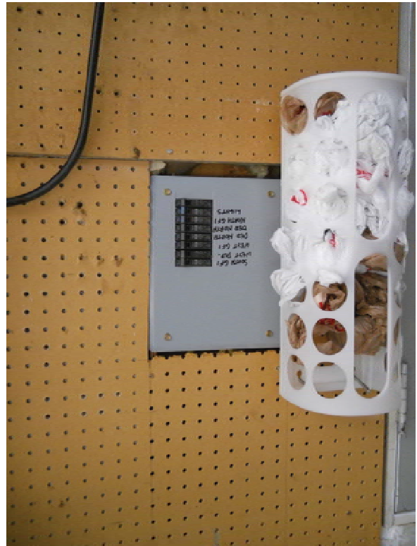
Interior electrical panel
