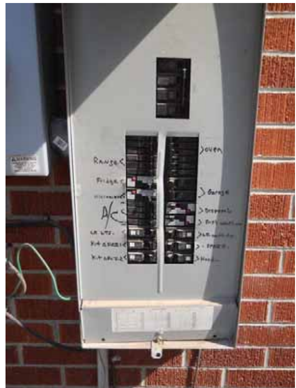
Exterior electrical panel
