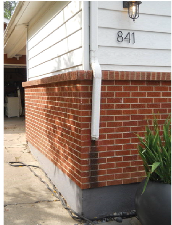
Downspout with missing extension
