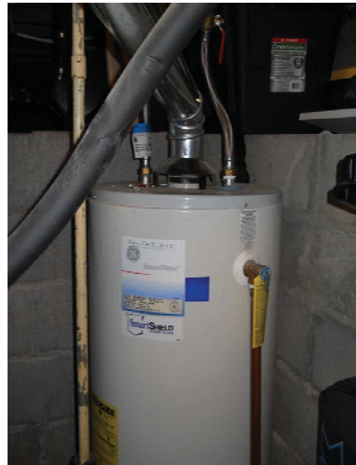
Hot water heater
