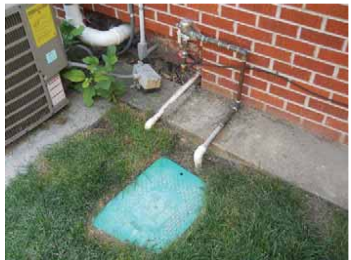
Unsecured electrical box at condensing
