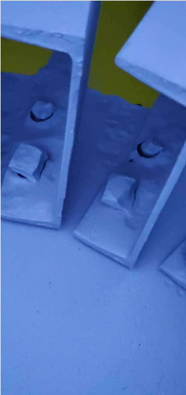
Bolt heads corroded away
