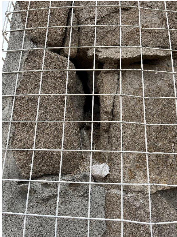
Photo 14: NW corner – mortar deterioration
