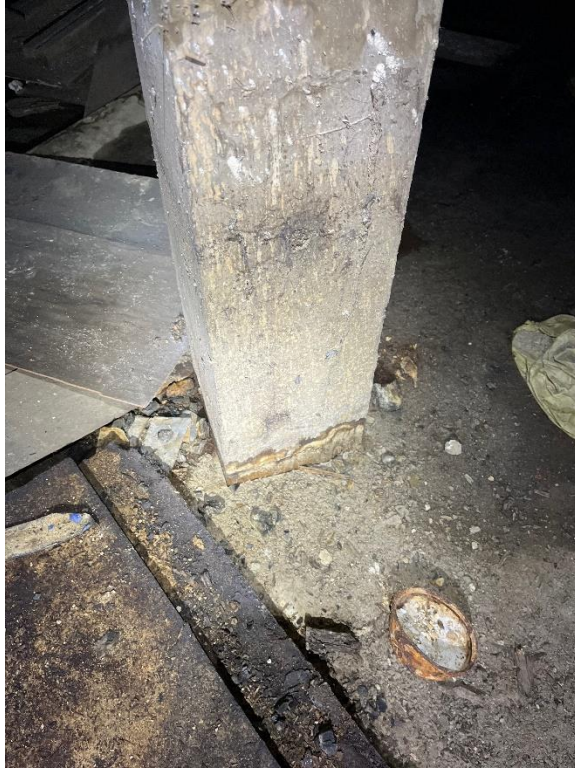
Photo 17: Timber framing – deteriorated post base
