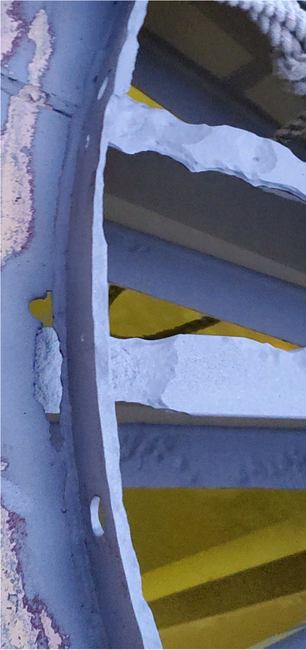
Metal loss on rafter and circular brace; hole in circular brace
