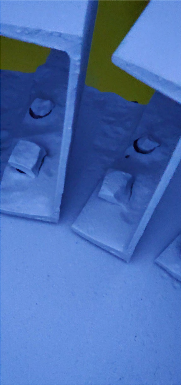
Bolt heads corroded away
